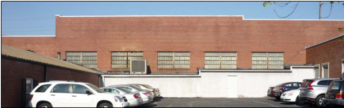
Photo 7: East Elevation Showing Original Windows. Lean-to additions and buildings at left and right are not part of the study property.
