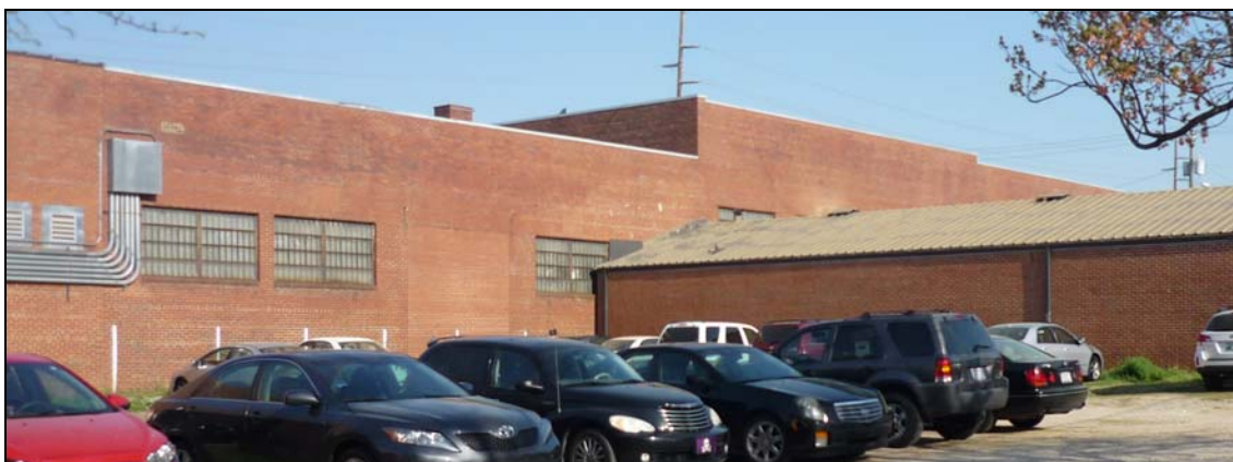
Photo 9: View of East Elevation Looking Northwest, Showing Chimney. One-story gabled building attached to the east elevation (at right) is a part of another property.
