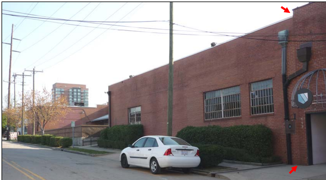
Photo 6: View of West Elevation, Looking North-Northeast. Cold joint in masonry wall and change in parapet height and coping at right denote the separation of 411 W. Morgan Street from 117-121 S. West Street (highlighted by red arrows).
